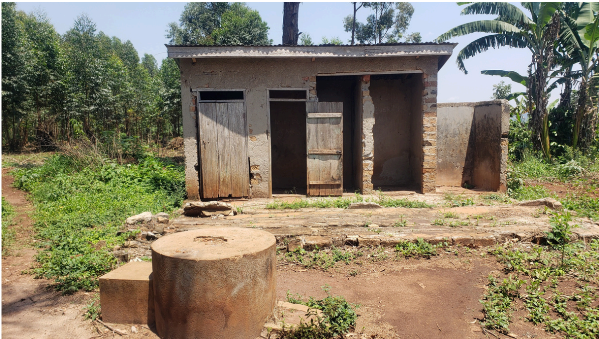
Fig 1: A section of the pit latrine that was decommissioned after it sank.
