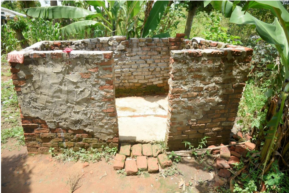
Fig 4: A photo of the bathroom that was renovated with a cemented floor taken on 22 nd October, 2024.
