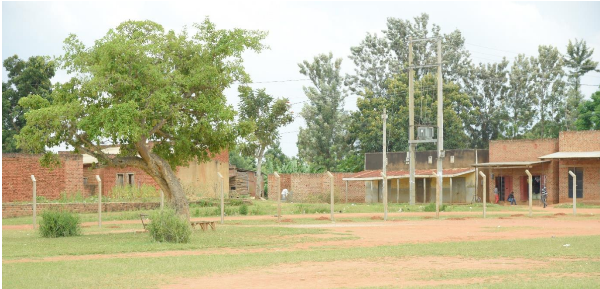
Fig.2: Some of the new fence poles in site at Nakisenyi Primary School (Photo captured on 23 rd October 2024)
