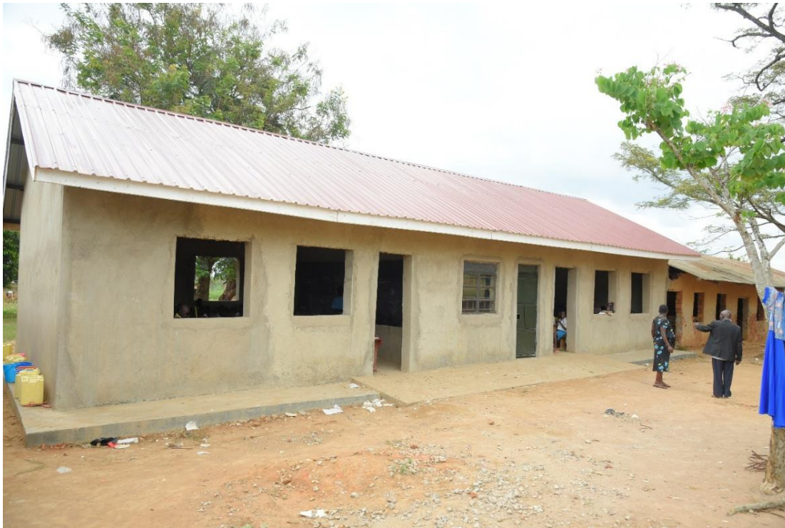
Fig. 1: The new classroom block at Nakisenye Primary School captured on 23 rd October 2024
