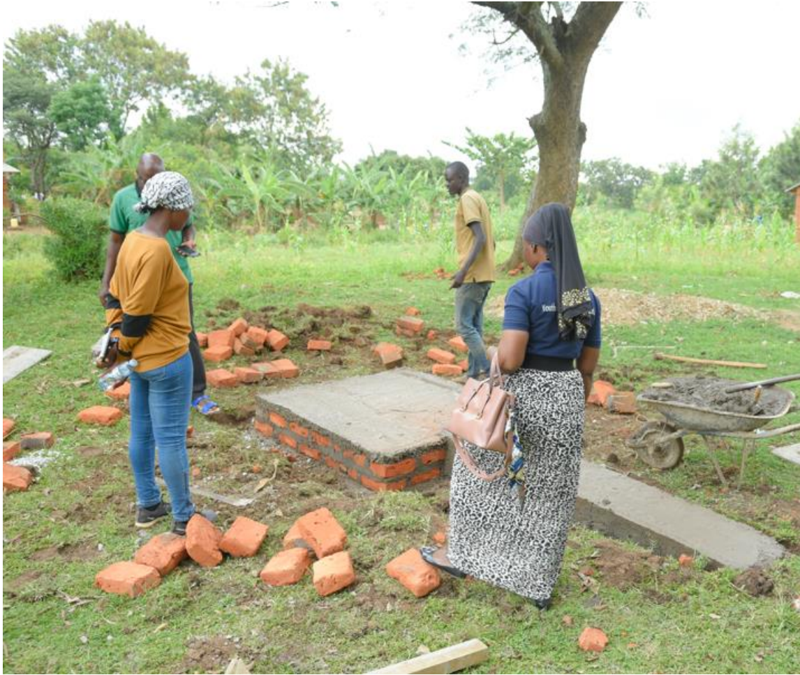
Fig.1: A new water source (tap) under construction at Lyama Seed School. (Photo captured on 23 rd October 2024)
