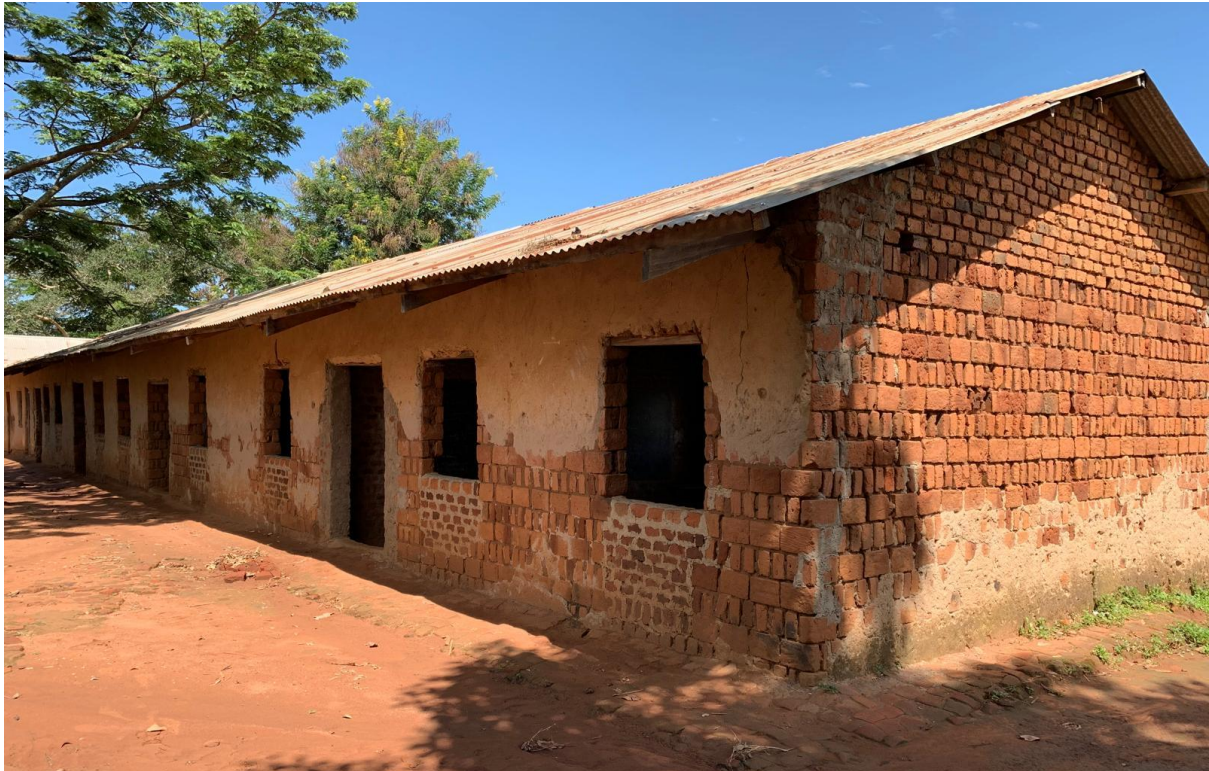
Old classroom block of Nakisenye Primary School, Lyama Town Council, Budaka District (Photo taken on 22 nd May 2024)
